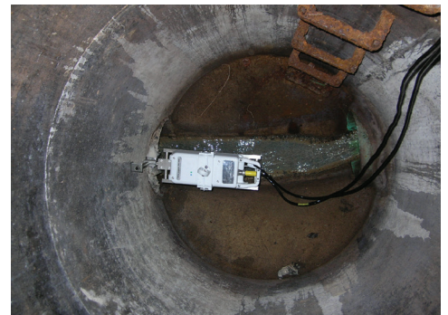
DDS Flo-Dar Sensor installed in a manhole
